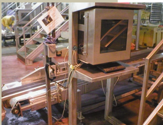
Quick-disconnect printheads are held in stainless-steel enclosures, top. Conveyors, middle, are set up to carry cases past the two printheads. Control components are housed in a stainless-steel cabinet, above.
